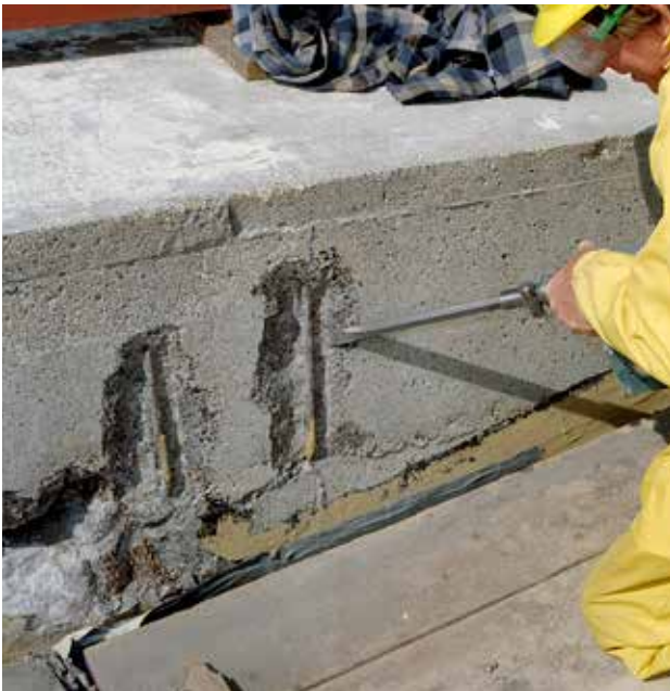
Damaged concrete structure
