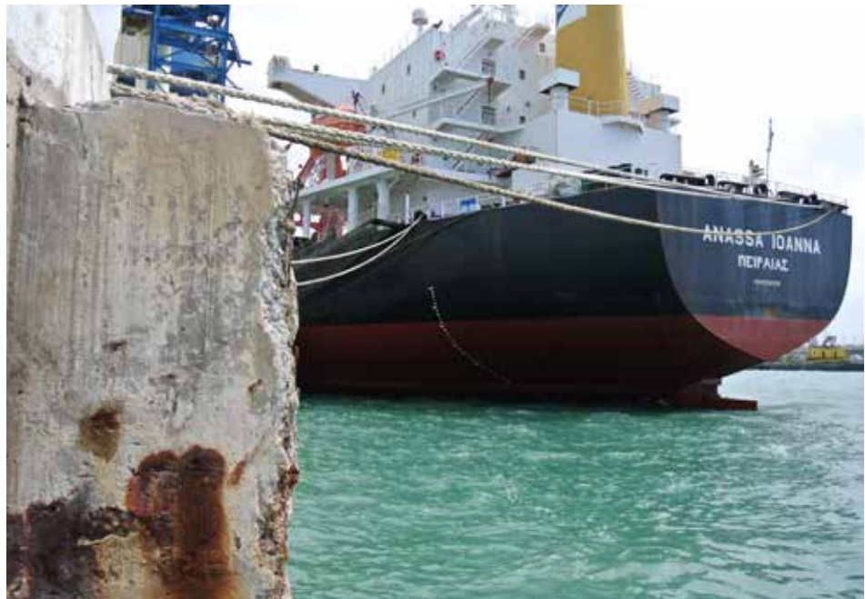
Reinforcing steel corrosion in a pier.
