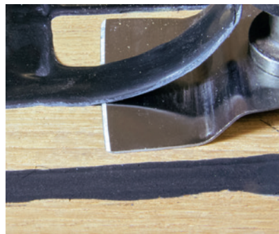
Fig. 38 Picture Removal overstanding Sikaflex®-290 DC PRO with a vibrating scraper power tool
