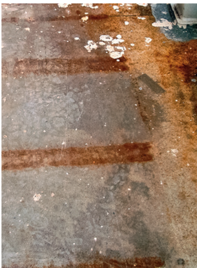
Fig. 2 Typical welds and weld splatter of a steel deck
