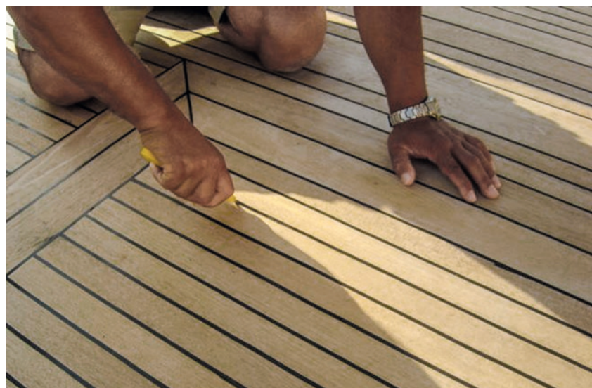
Fig. 23 Using a craft knife to cut along the part of the joint to be removed
